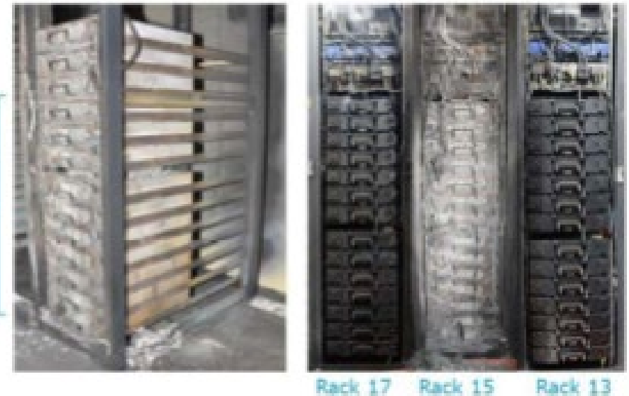
Figure 4: All modules in Rack 15 were severely damaged by thermal runaway while leaving nearby racks mostly intact (Image credit: APS) [1]
