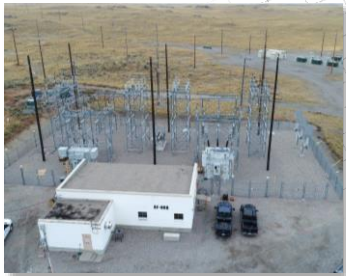
Dedicated R&D Substation
