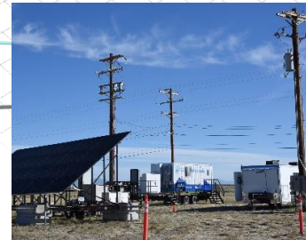
Mobile Command Center, PV Super Array, and Wind Turbines
