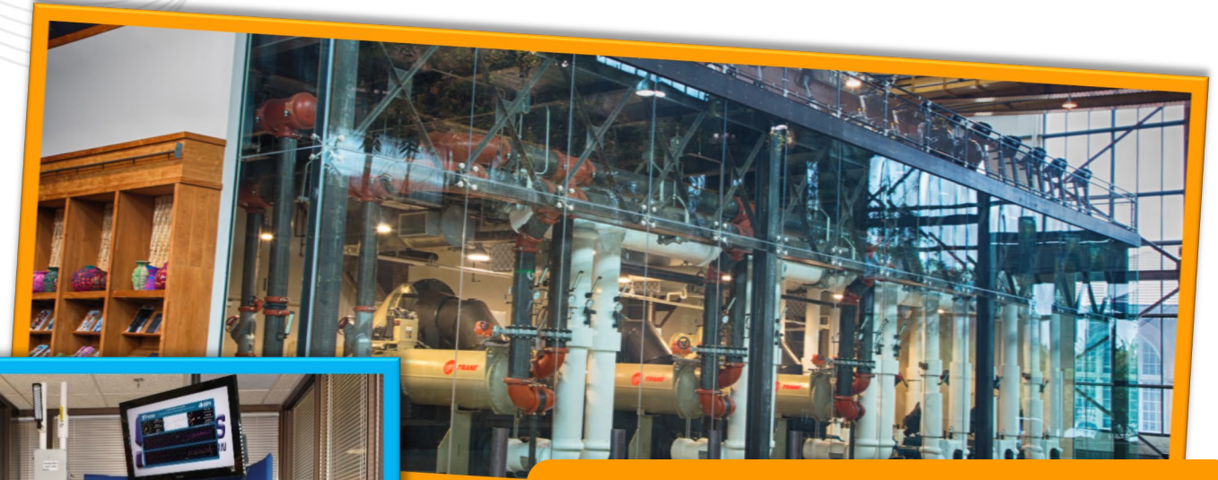
Chiller at Philadelphia Navy Yard
