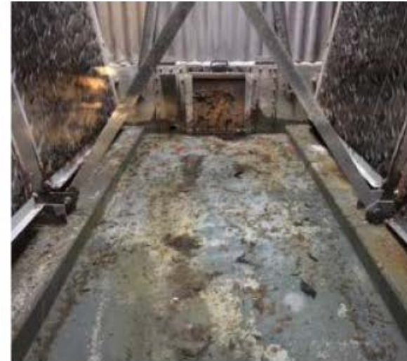
Cooling tower interior pan
